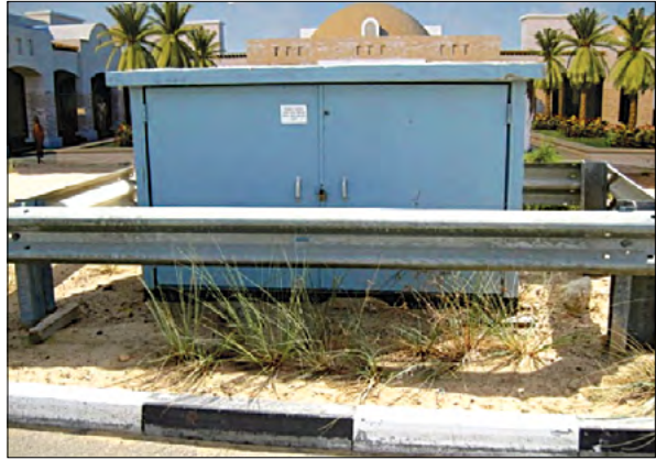
1.4.3A.1 Vertical mounted link box with steel crash barrier protection on the side of a road.
