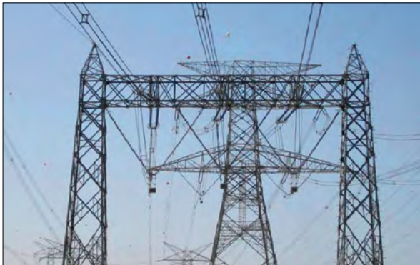
c. 400/132kV Gantry Tower
